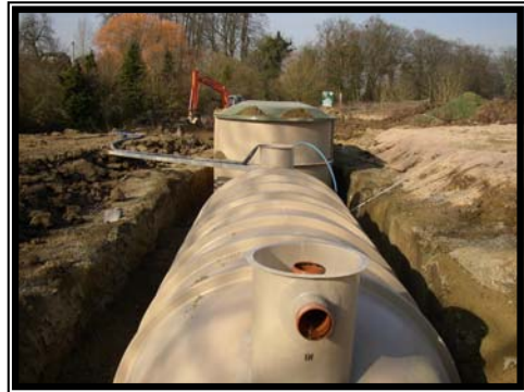
A 300 PERSON TREATMENT PLANT INSTALLATION FOR A HOTEL AND LEISURE COMPLEX
